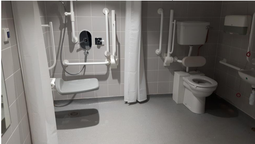
Figure 40: New Shower facilities in Block F (4 independent units)
